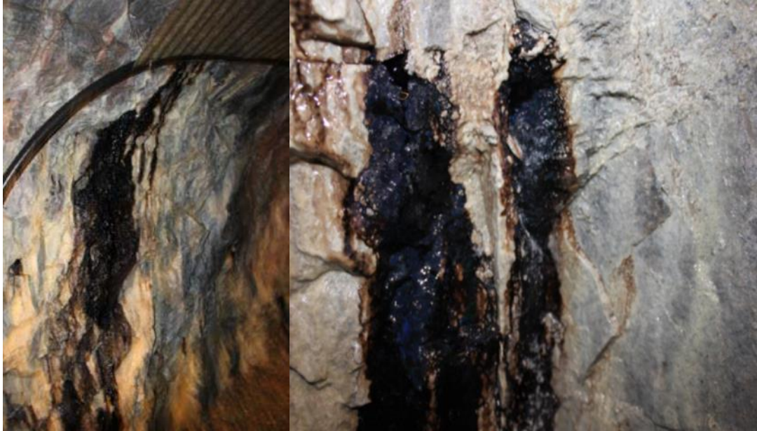
Fig.4: Ytterby black substance (YBS) seeping from fractured bedrock in tunnels leading to the main shaft of the Ytterby mine.
